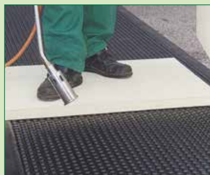
Heat insulations in panels
